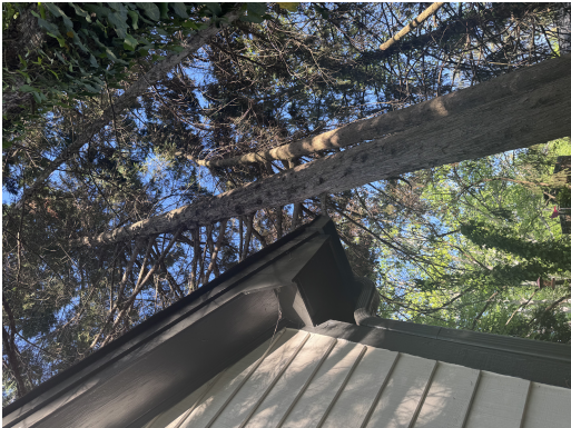
Large trunk resting directly against the roof corner and chimney.
