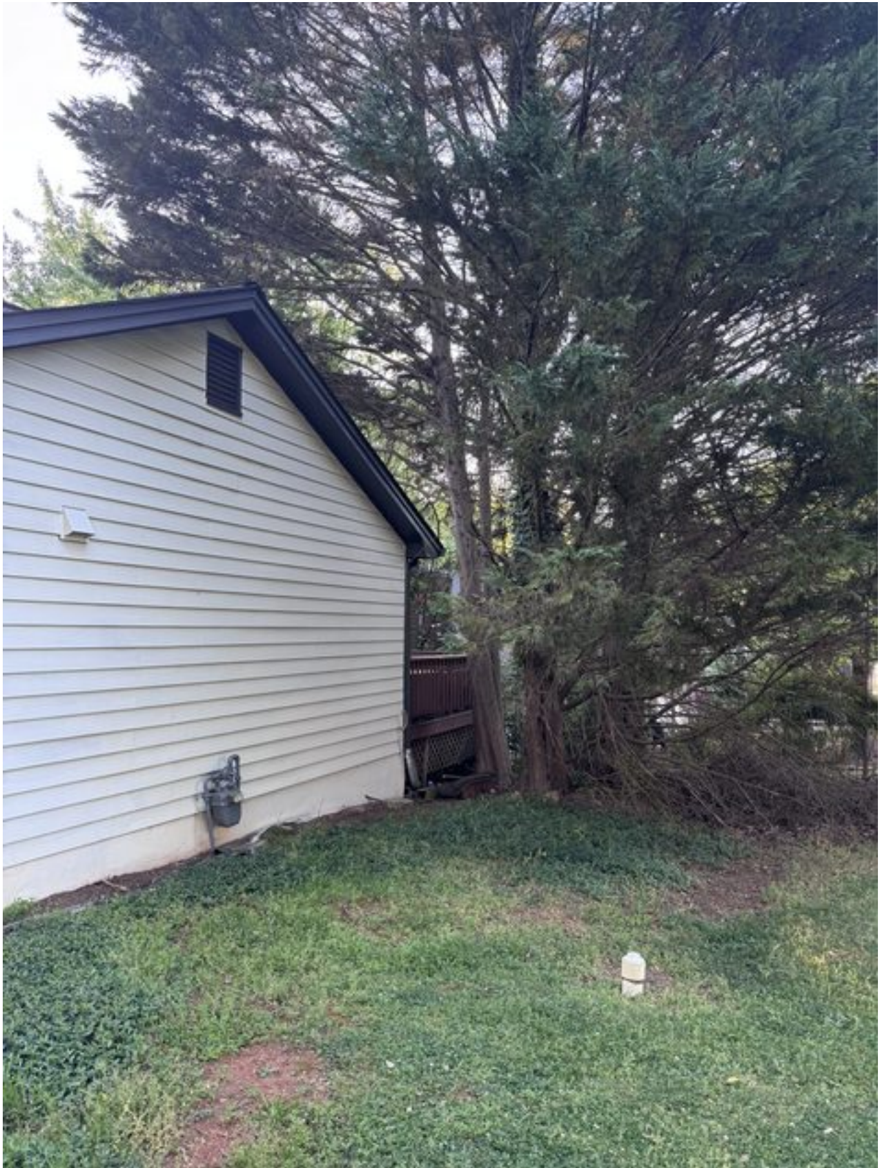
EXHIBIT E — Photo 1 of 11: Aerial/elevated view — Leyland Cypress cluster directly over the roofline at 275 Truehedge Trace. The canopy extends over and onto the roof of the primary structure. Trees are well within the 8-ft. minimum clearance from the structure required by industry standards and referenced in Tomahawk Estimate #13801.
