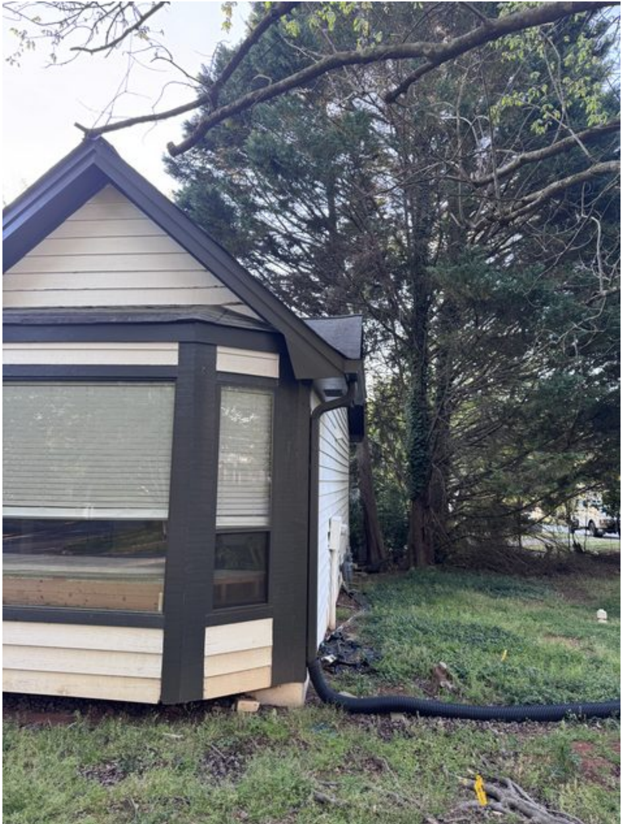
EXHIBIT E — Photo 9 of 11: Full side-elevation view — Leyland Cypress alongside and over the structure.
